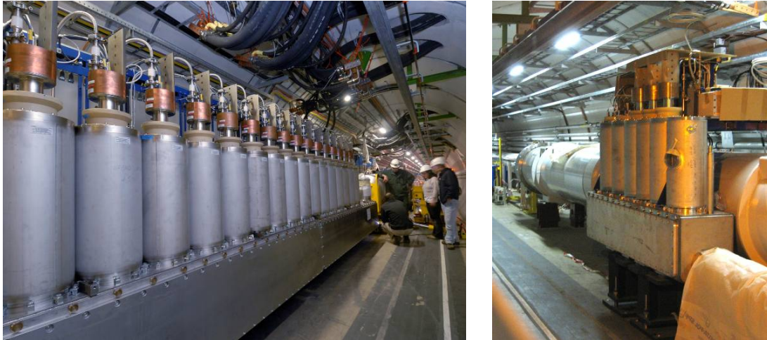
FIGURE 3. pictures showing the DFBA powering one of the sides of sector 7-8 (left) and a DFBL powering one of the standalone magnets (right) installed in the LHC tunnel
