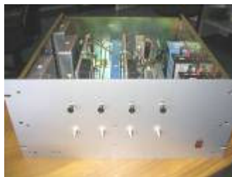
Figure 11.1.4: BPM subsystem located in the hall
