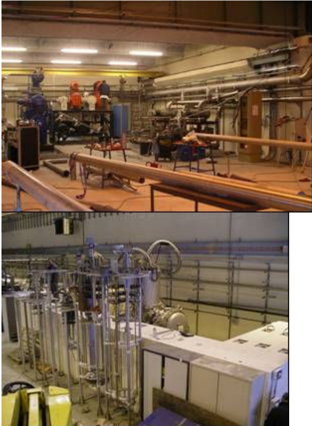
Figure 10.6. Re-installation of the helium compressor and vacuum pumping system (left) and the CryHoLab area (right).
