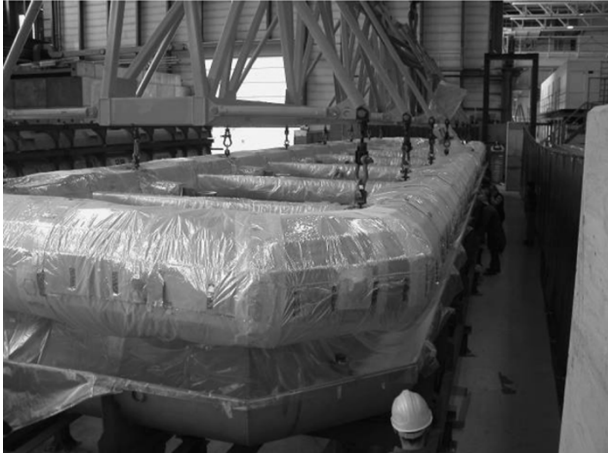
Fig. 3. The cold mass held by the high inertia lifting frame being lowered down in the vacuum vessel. Gaps between the vacuum vessel and the superinsulation are controlled.
