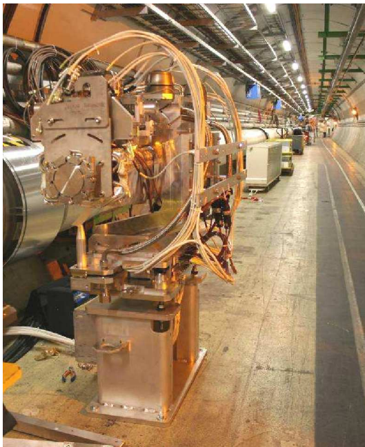
Figure 3: Photograph of LHC collimator installed on its base-support assembly (base-support and quick plug-in).
