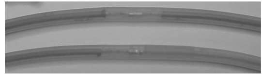
Fig. 10. Examples of HV cable connections.
